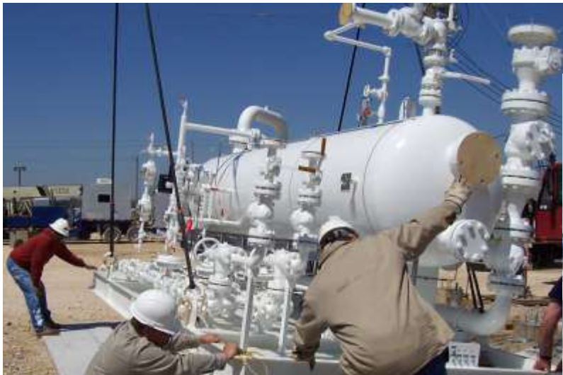
Valves for a gas gathering and transportation station
