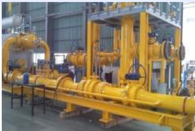
SAMRA POWER STATION PHASE-III, SIMPLE CYCLE PROJECT
