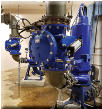
Swing Check Valves Hendersonville, TN
