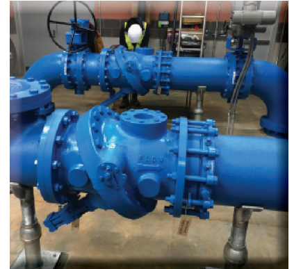
Tilted Disc® Check Valve & American-BFV® Butterfly Valves Lexington, NC
