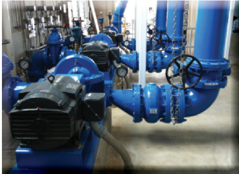
Air Valves, Silent Check Valve and American-BFV® Butterfly Valves Princeton, IL
