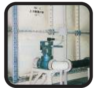
Emergency shut-off valve
