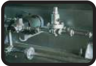
Pressure reducing valve for oil
