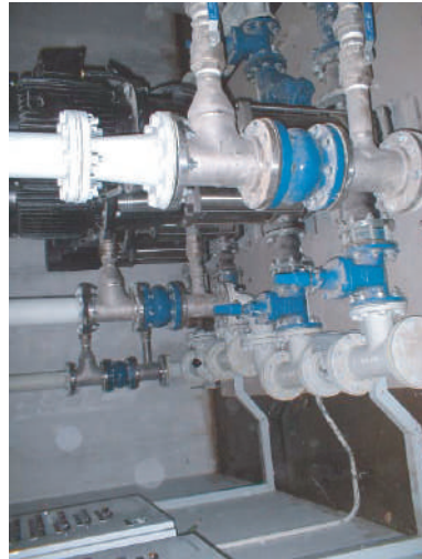
Side view of pump room.
