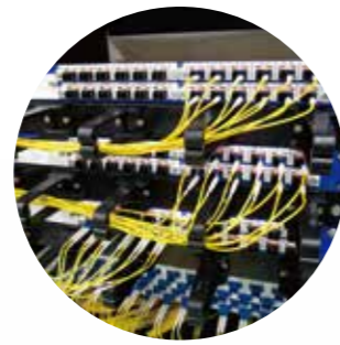
Telecommunication Infrastructure Components
