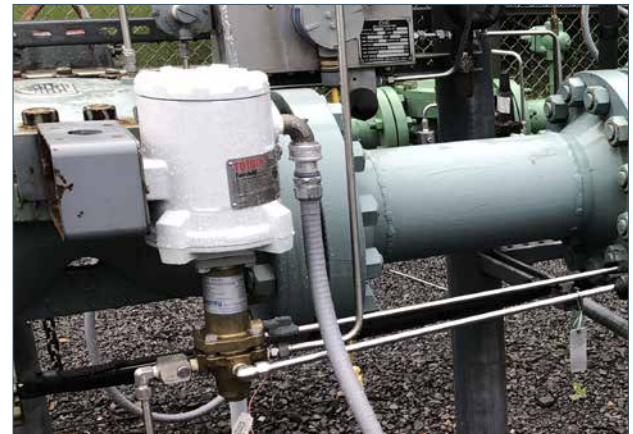
PAX 1 installed in pressure control and metering stations for natural gas distribution
