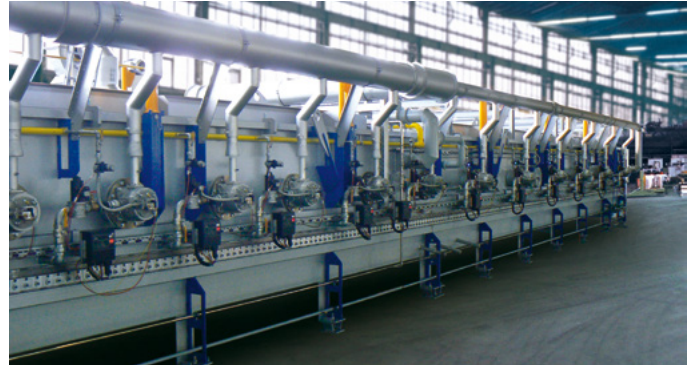
Tailored blank furnace
